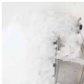
Ice piles up below the output fitting, eventually obstructing the ice level sensor "eye".
